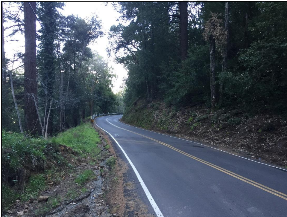
Figure 1.4. Narrow windy roads are common throughout the County, which is a concern for emergency response as well as evacuation.
